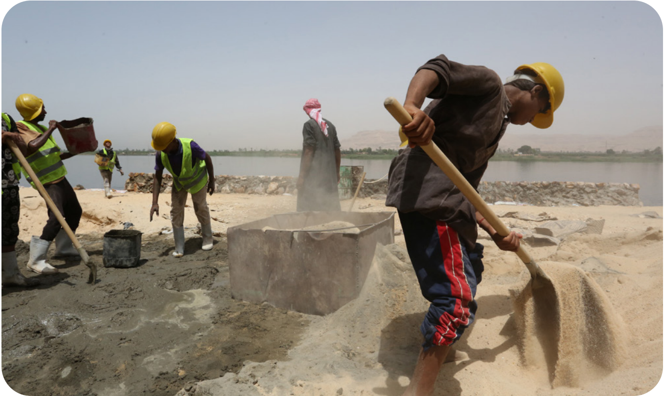
A project in Luxor, Egypt, creating short-term employment opportunities for unskilled and semi-skilled workers and providing access to basic infrastructure services. Photo: Dominic Chavez/World Bank
